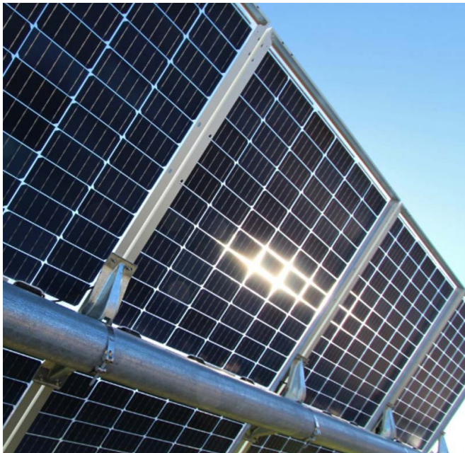
IMAGE OF A BIFACIAL SOLAR PANEL SYSTEM
